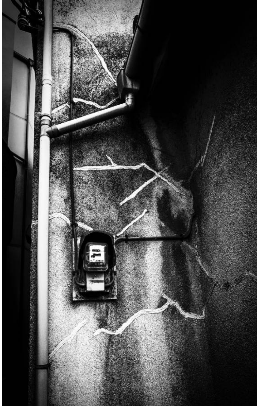
Meg Hewitt Cracks in the wall, Tokyo, 2016 Gelatine silver print
